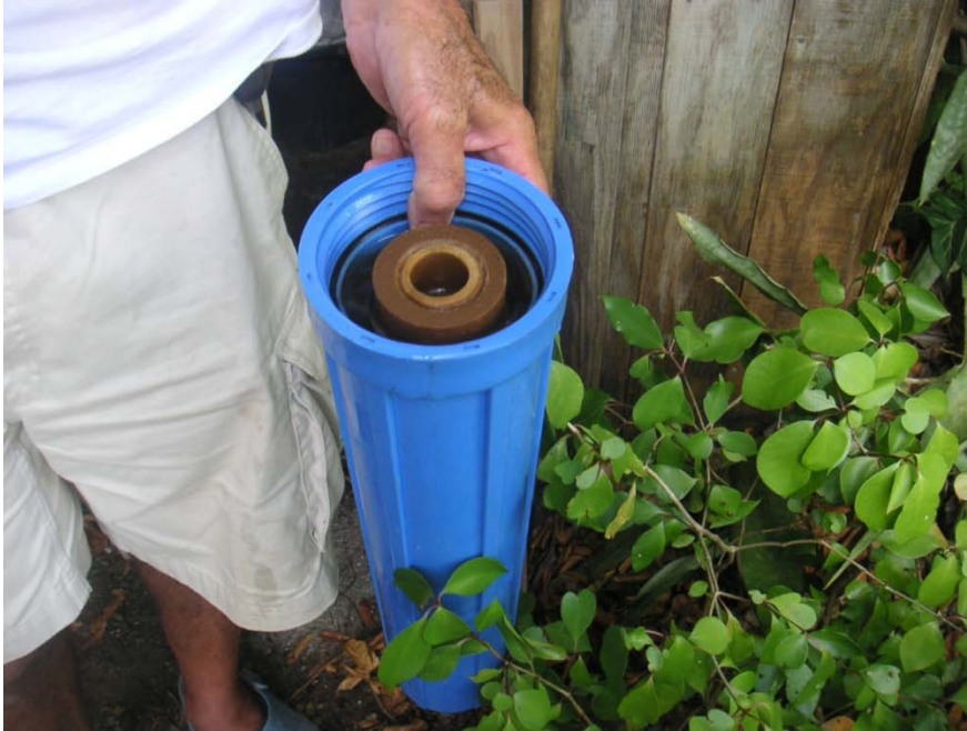
Dirty filter and dirty water – in first chamber.
